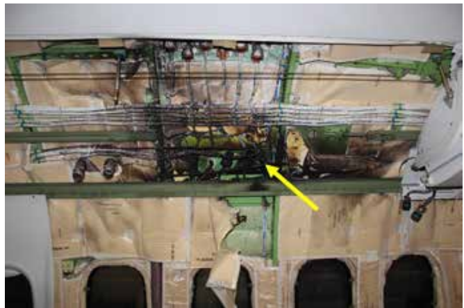
Figure 2. Area of heat damage at row 14 of the occurrence aircraft, shown with left cabin wall upholstery removed (arrow indicates electrical connector 9811-J711)
