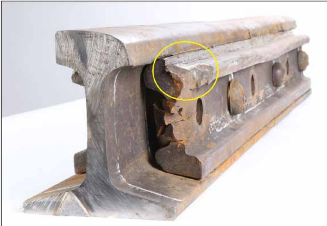
Figure 8. Gauge bar and bolt hole with wheel flange impact damage on the corner of the joint bar (circled)
