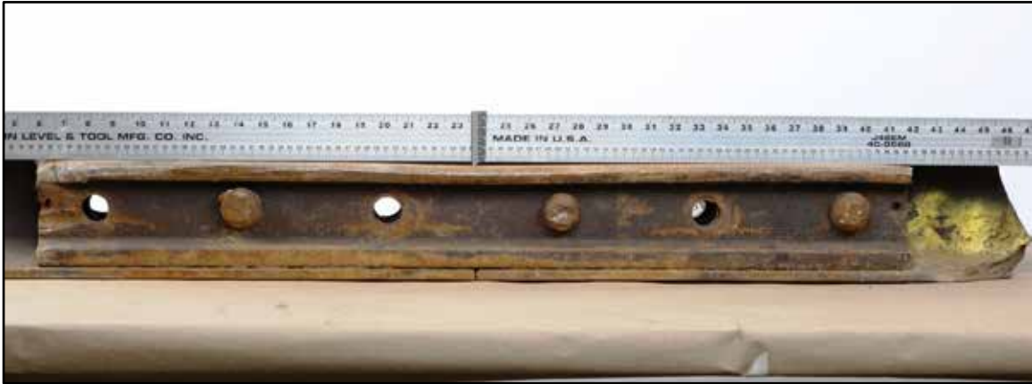
Figure 6. Gauge joint bar with missing bolts
