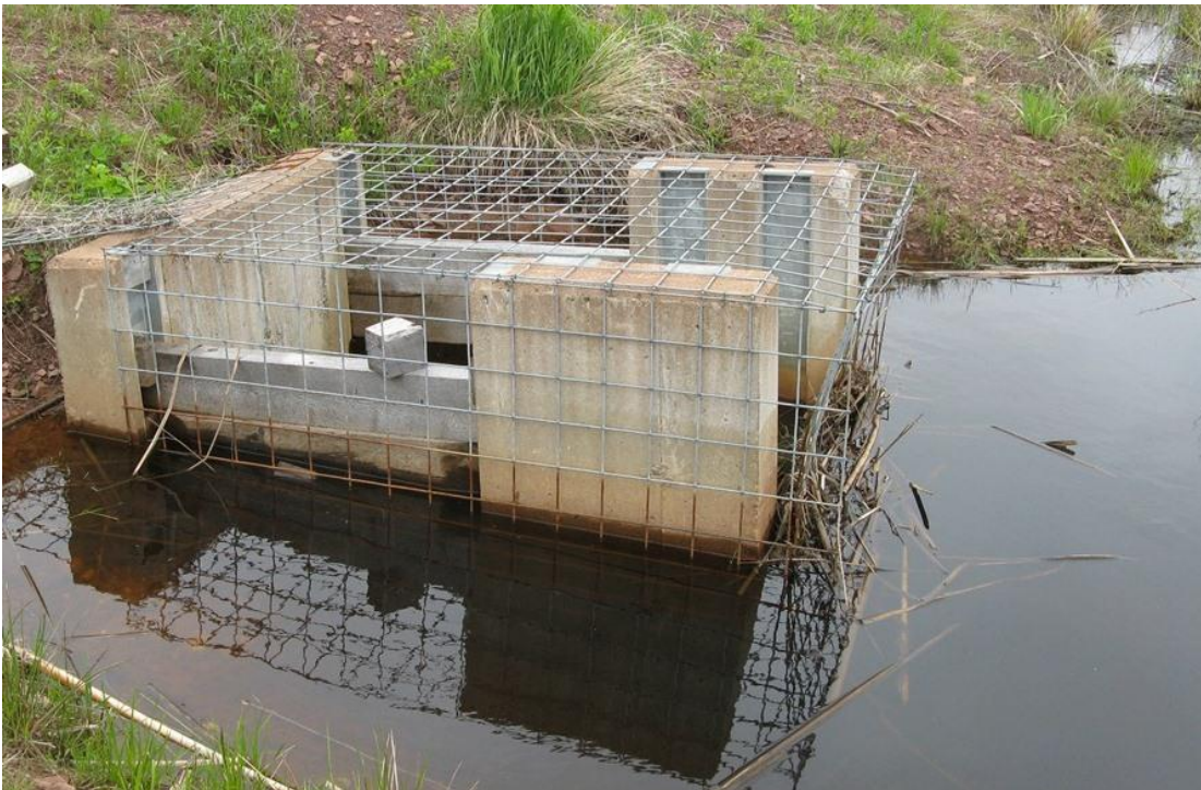
Figure 15: Example of a typical control structure used to regulate water levels within an impoundment. A wire cage is applied to reduce plugging from beaver activity. Photo: C. MacKinnon © Environment and Climate Change Canada, 2013
