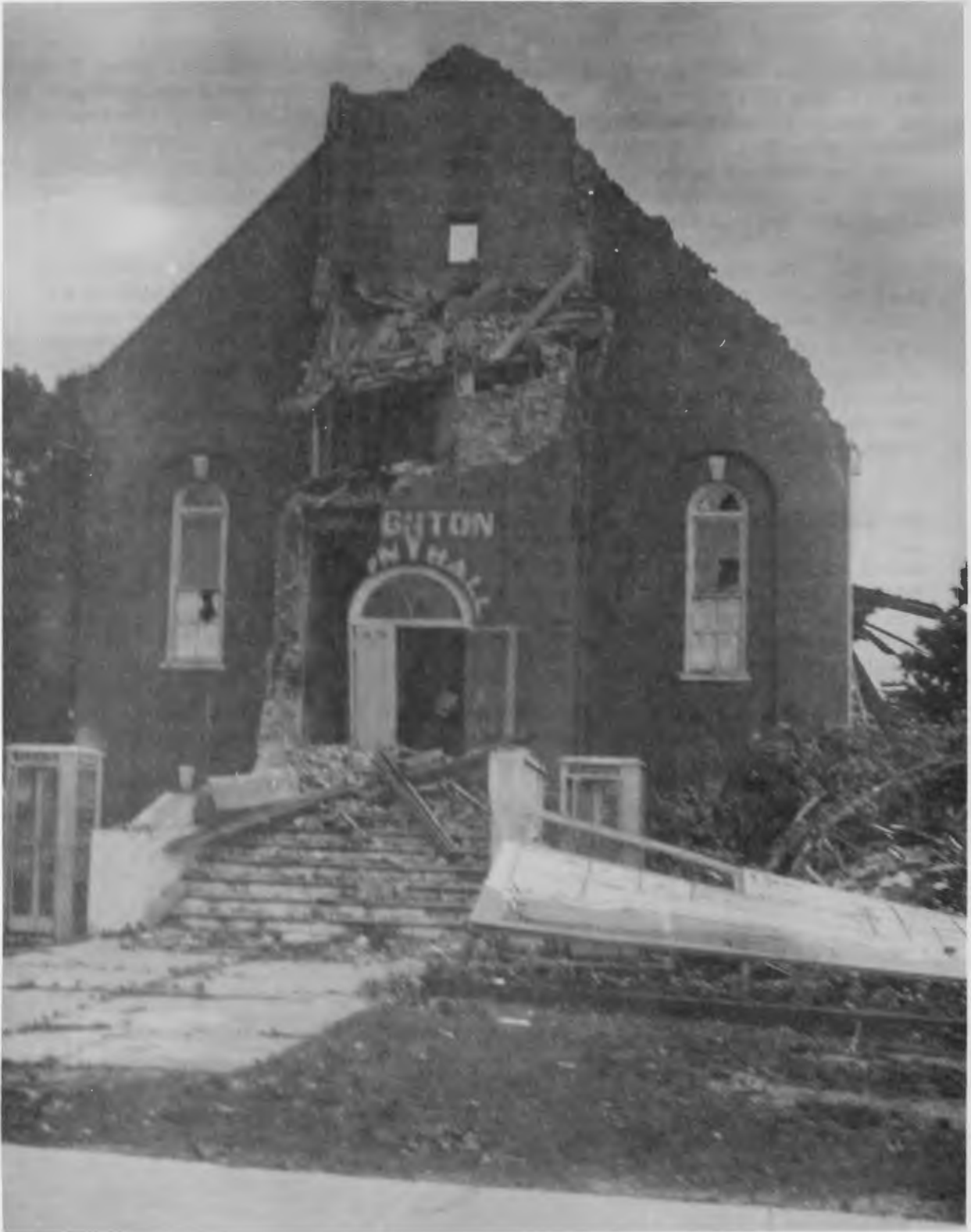
Typical damage caused by the tornado which struck Brighton, Ontario on July 13, 1973.
