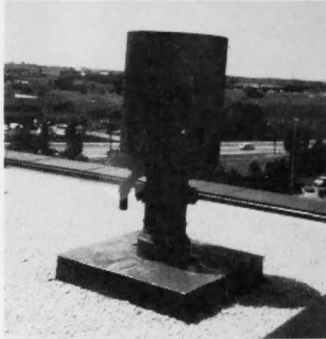
The radome base contains one of the roof's strangest objects — an ugly brown container resembling a dinosaur's drinking cup. It's used as a spare exhaust for the boiler room.
