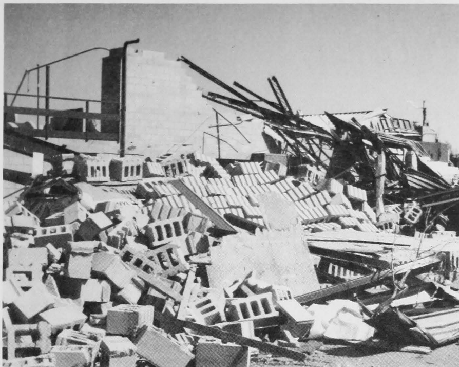
Cinder block concrete bricks from a Barrie industrial building scattered far and wide give the area the look of a battlefield.
