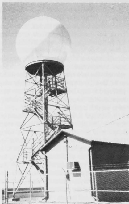
Installing the New Brunswick weather radar. The only real snag occurred when the crane operator had trouble removing the radome because it was bolted down.
