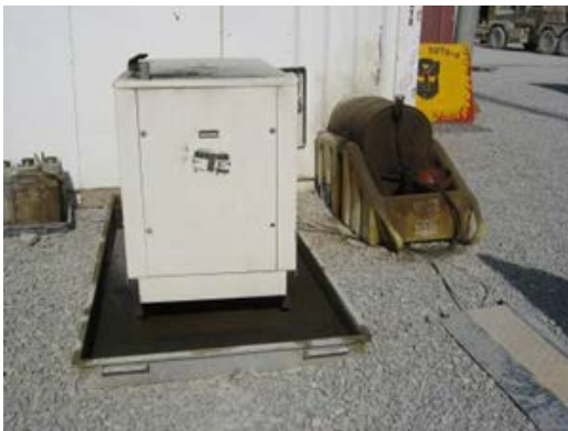
Figure 5: Secondary Containment for a Generator
