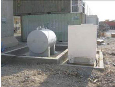
Figure 6: Concrete Secondary Containment Dykes for Fuel and Generator
