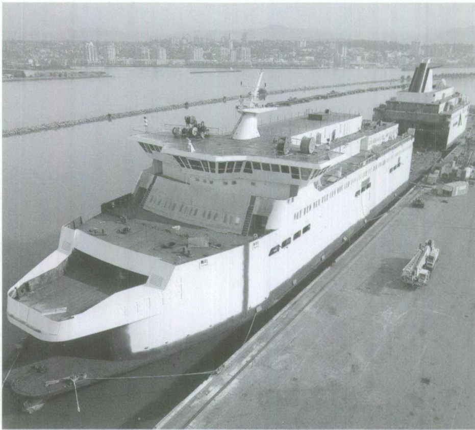
The joining of superstructure and hull during construction of the B.C. Ferry Corporation's new S-Class Ferry, M.V. Spirit of British Columbia (Courtesy of Avcom International Ltd.).
