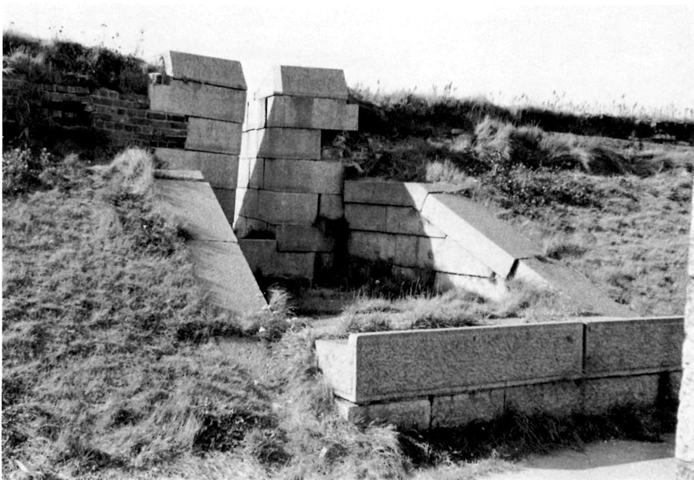
37 Detail of one of the west ravelin embrasures, 1971. The granite embrasures in the west ravelin were unique in the Citadel. There were originally four of them, two in each face. Two now survive. ( Photo by author. )
