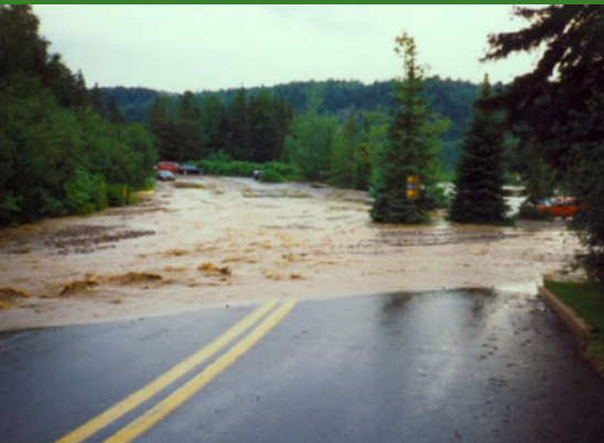
Figure 1: A flooded road at La Mauricie National Park. To avoid situations like this in the future, the Park is installing culverts designed to handle peak water flows seen every 50 years.
