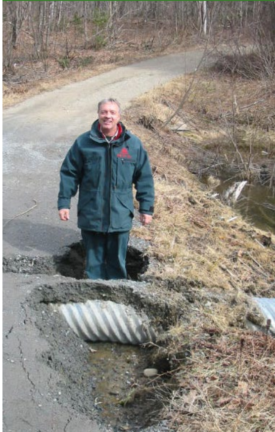
Figure 5: Yves Marcouiller inspects a failed culvert in La Mauricie National Park. When culverts become blocked or are too small to handle peak flows, the water erodes the gravel, creating a hazard to the public and sometimes covering fish spawning areas with sediments.
