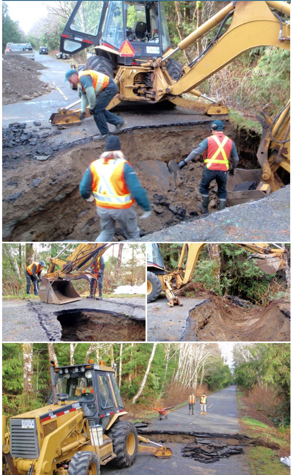
Figure 11: Parks Canada Team Members replace a culvert at Pacific Rim National Park Reserve. Geomatics Infrastructure maps will enable staff to share their corporate knowledge to plan for risks to employee safety (e.g. by identifying buried cables), built infrastructure, ecological integrity, cultural resources and Aboriginal values. (Photos: J. McIndoe, Parks Canada)
