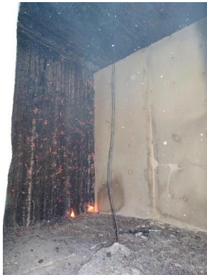
(e) Wall A (partial), Wall D and ceiling at 150 min
