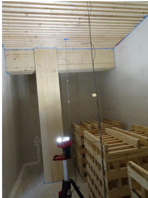
Figure 26. Fully exposed uneven NLT ceiling, Glulam beam and column for Test NLT-2.
