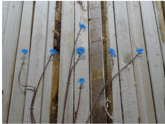
(a) Holes drilled from exterior side of NLT and sealed with 3M Fire Barrier sealant
