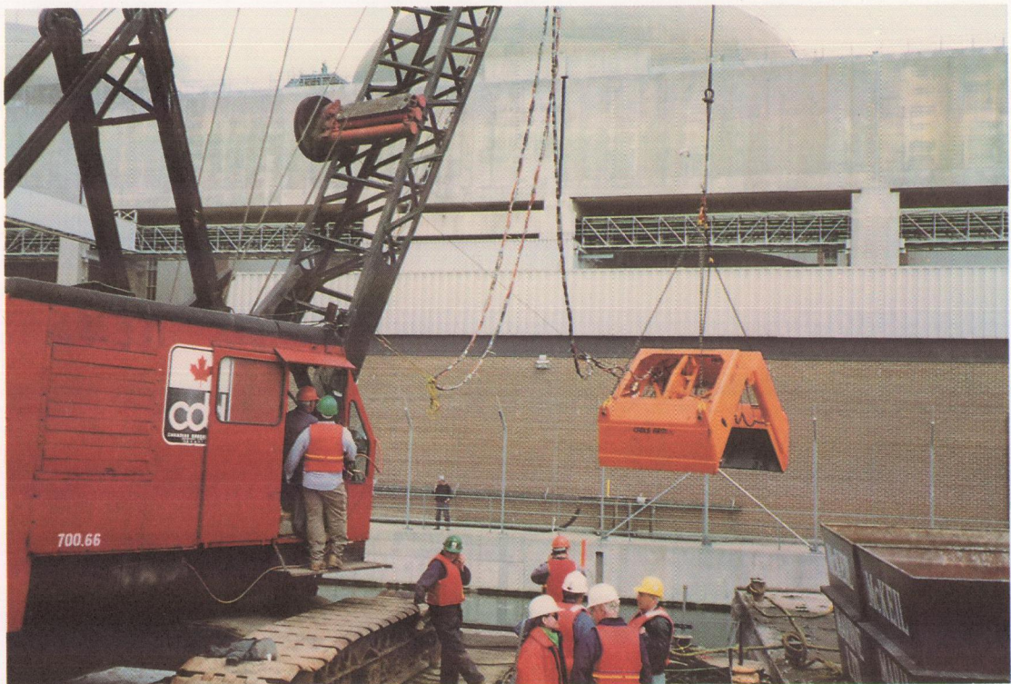
Cable Arm commercial use at Pickering.
