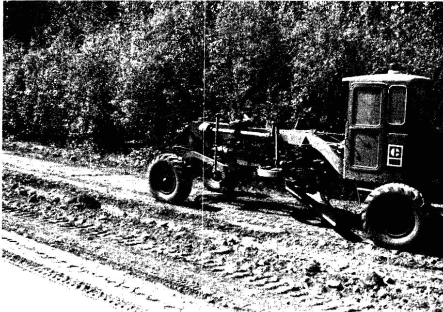
PLATE 6 Road grader clears a 4 m swath of vegetation. Cleared area in this picture is approximately 8 m wide, but it approaches 12 m wide in other sections of this highway. Robert Campbell Highway, km 56.
