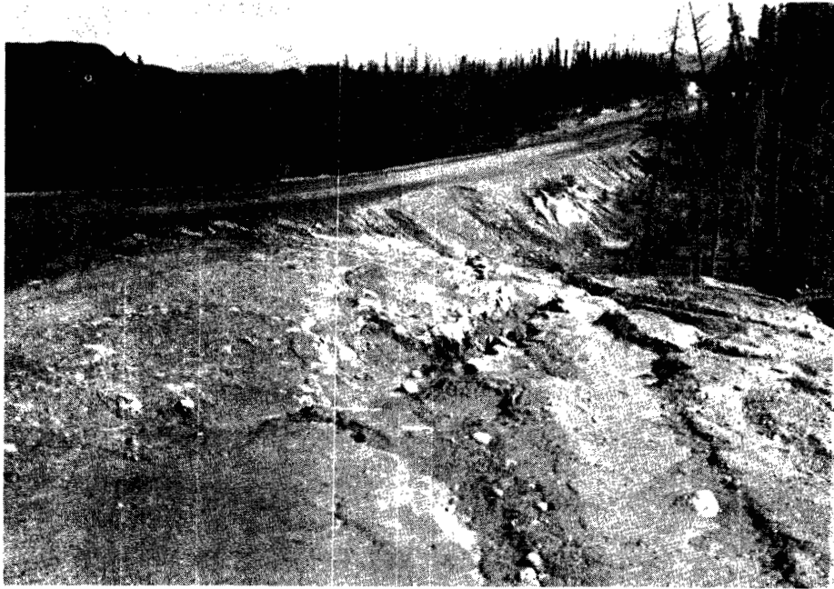
PLATE 10 Gully erosion silty, soil. Robert Campbell Highway, km 100.
