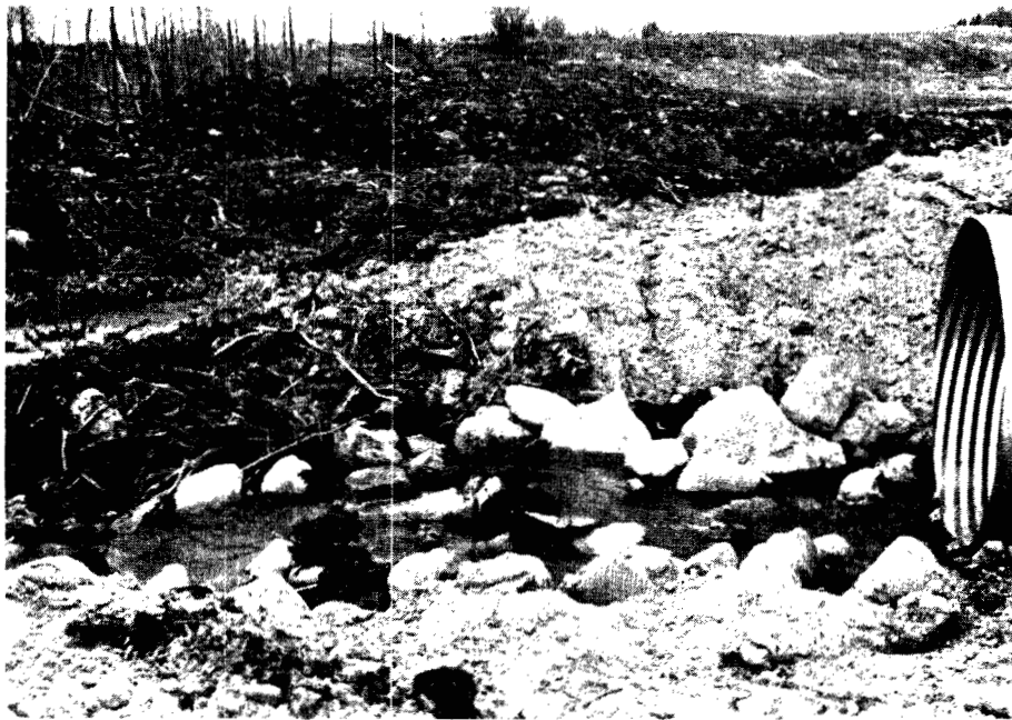
PLATE 57 Minor stream crossing, note extensive destruction of shorelands. Alaska Highway, km 1501. Section being reconstructed.
