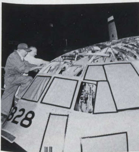
EDMONTON - Repairing damaged Canadian Armed Forces C-130 Hercules transport at Northwest Industries Limited.
