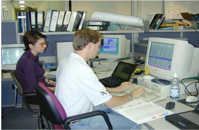
Figure 51: The command center is based on PC technology and easily located in an office environment.
