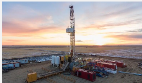
Test drilling rig, DEEP Earth Energy Production’s geothermal facility, near Estevan, Saskatchewan.
