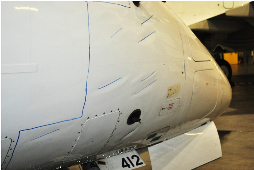
Figure 2. Wrinkled skin on the right side of the nose (blue dry-erase marker added for clarity) (Source: TSB)
