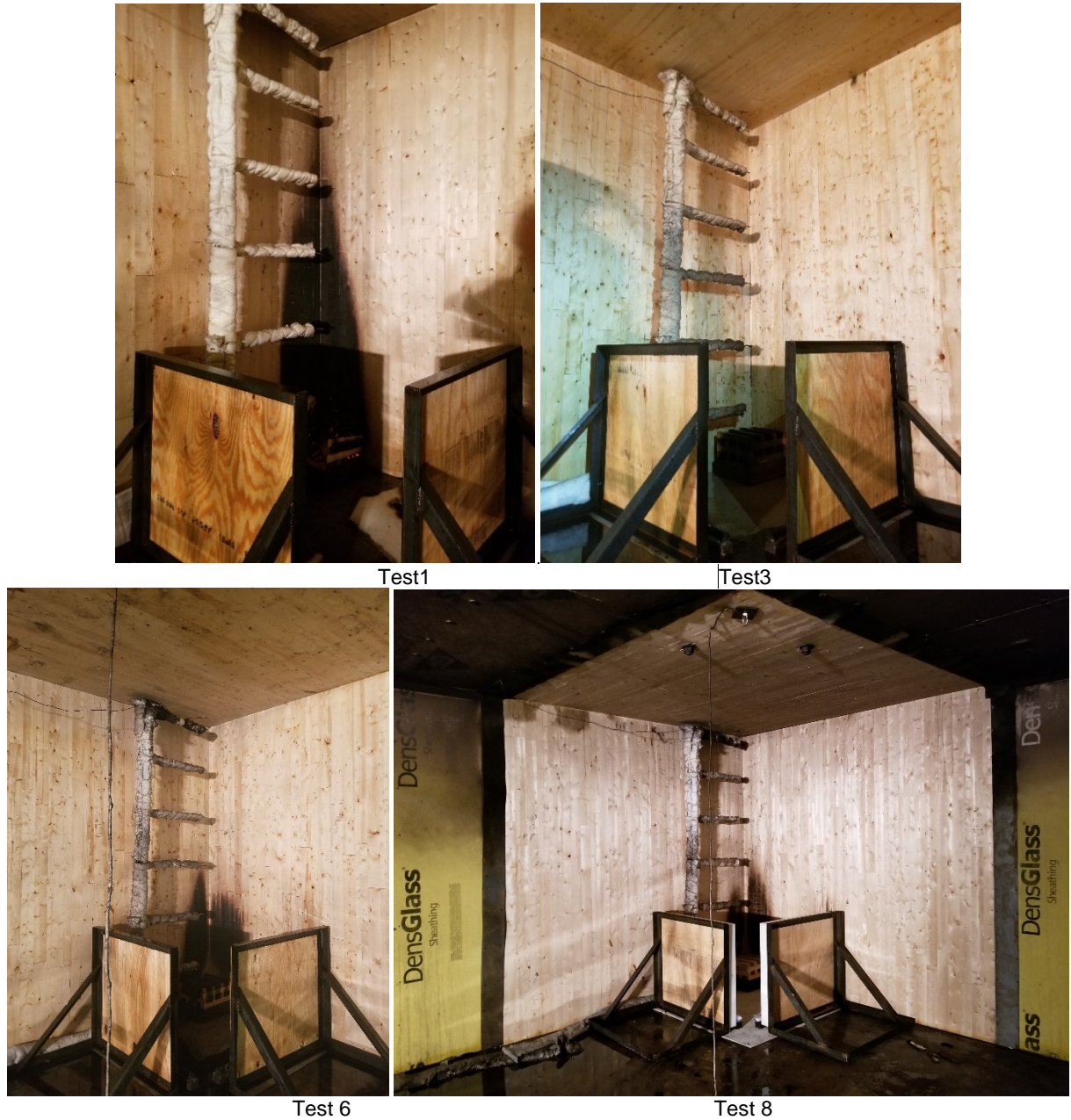
Figure 36 Fire damage on the CLT panels
