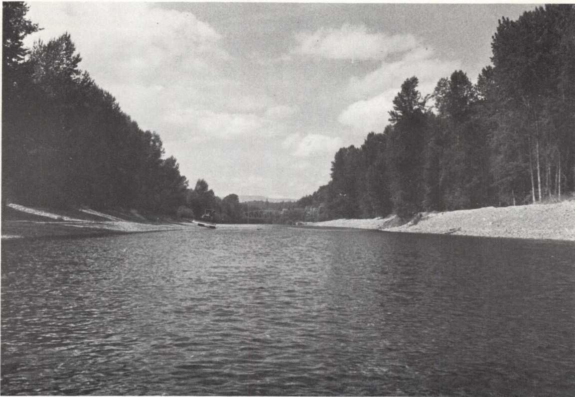
Section of river downstream of Island Highway bridge (background of photo) with excellent chum gravel. Note bulldozer and dyking.
