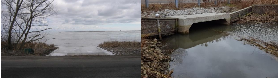
a) b) Figure 8. a) Aquatic wildlife culvert on the east side of Highway 59 (Causeway) connects the Inner Bay to the Big Creek Unit (2016), b) Aquatic wildlife culvert on the Big Creek Unit side, Big Creek National Wildlife Area, 2018.
