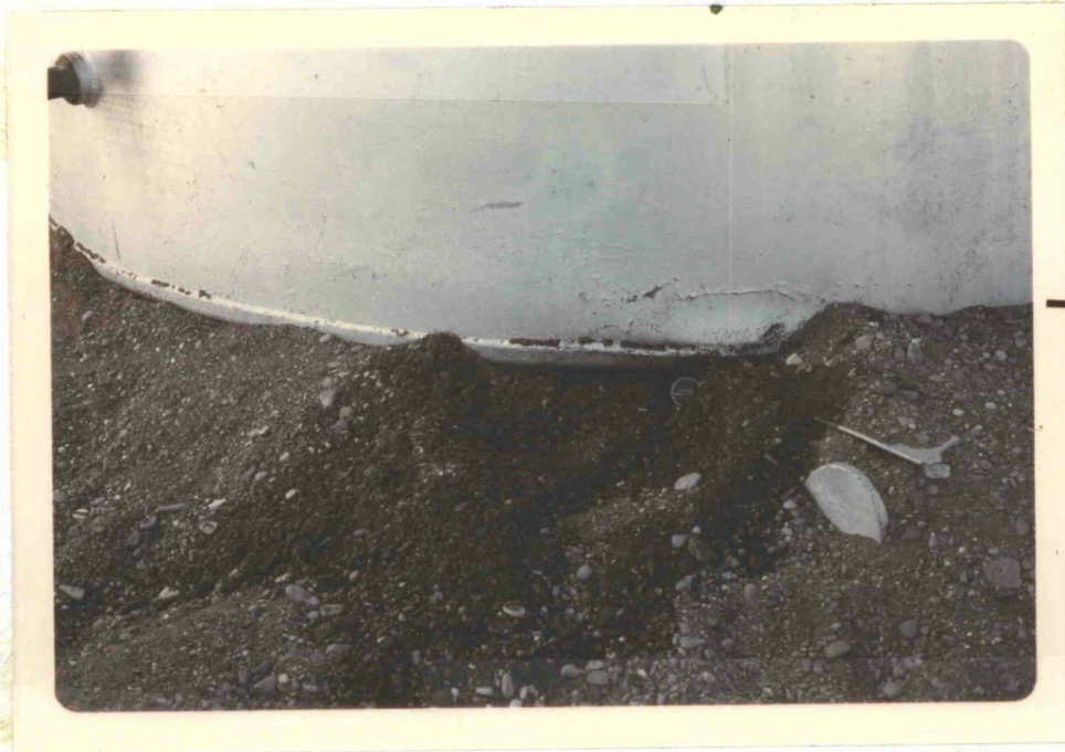
A small leak in one of the fuel tanks. Damage was caused during erection.
