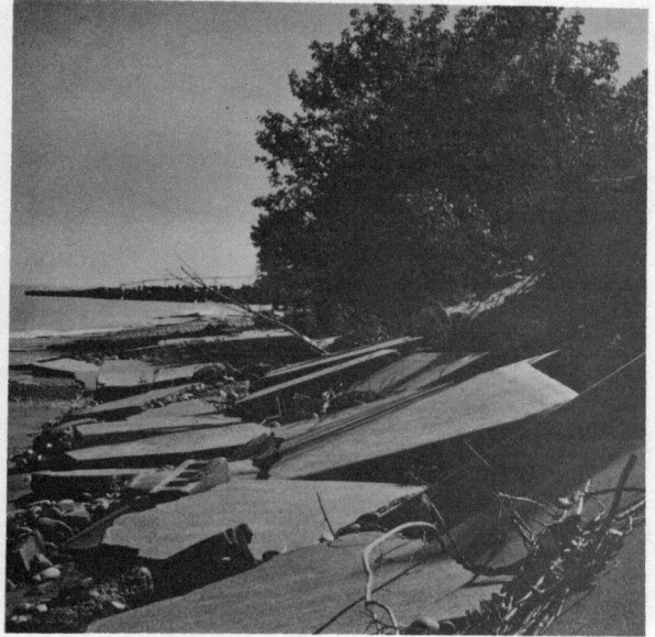
Concrete walk undermined and collapsed by wave action
