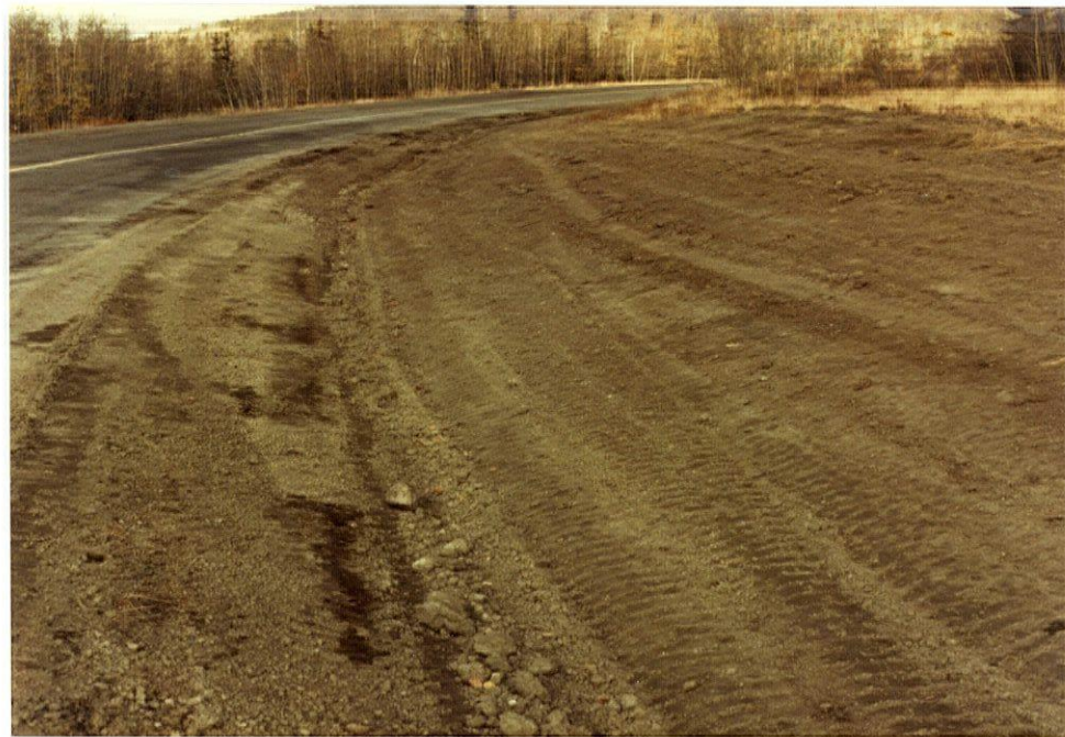
PLATE 84 - Blading, if necessary to restore drainage systems, should not expose large areas (km 1547, Hwy. 1).
