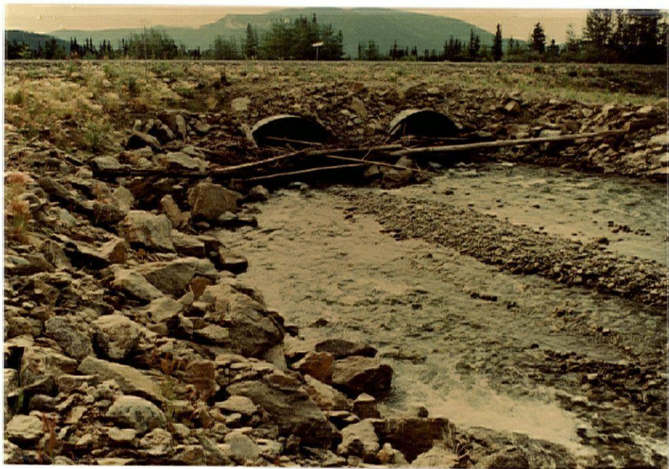
PLATE 72 - Debris will affect the capacity of the culvert to pass water, which is particularly important during periods of high flow. Improperly maintained culverts are a threat to the stability of the road embankment (Km 29.6, Hwy. 5).
