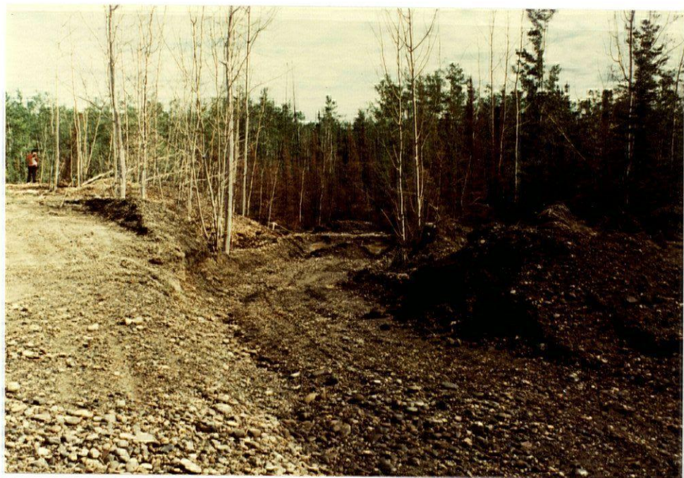
PLATE 76 - Surface runoff from a calcium chloride stockpile site is affecting the nearby vegetation (km 38.9, Hwy. 11).
