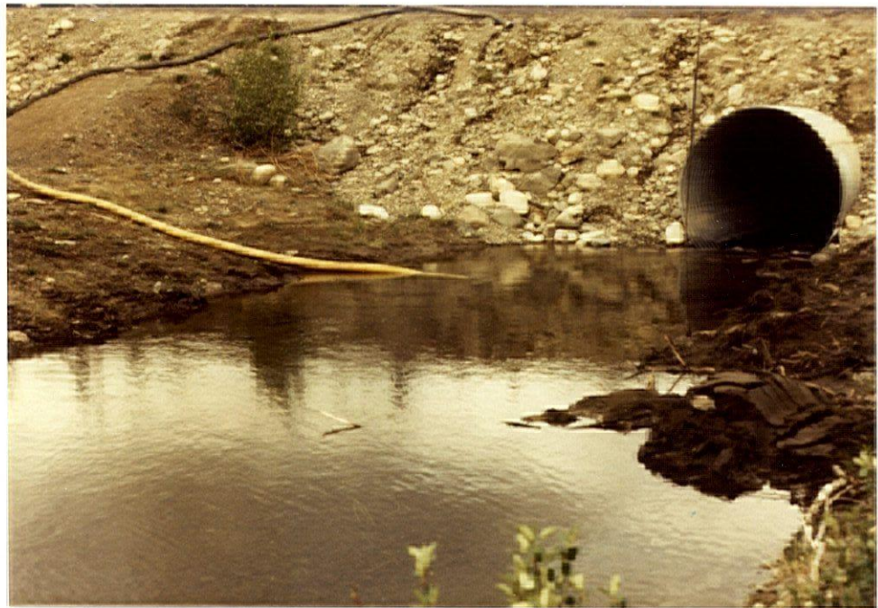
PLATE 78 - The spoil from this sump was deposited into the stream on the right hand side of photograph. If sumps are necessary, the spoil material should be deposited in a stable location above the high water mark (km 128.3, Hwy. 2).
