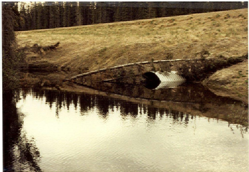
PLATE 70 - Debris plugging this culvert blocked fish passage and flooded off-right-of-way vegetation (km 1411, Hwy. 1).
