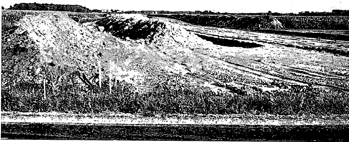
Photo 9. Topsoil and subsoil are piled along a pipeline right-of-way across productive corn fields in eastern Ontario. V. Kirkwood, Agriculture Canada
