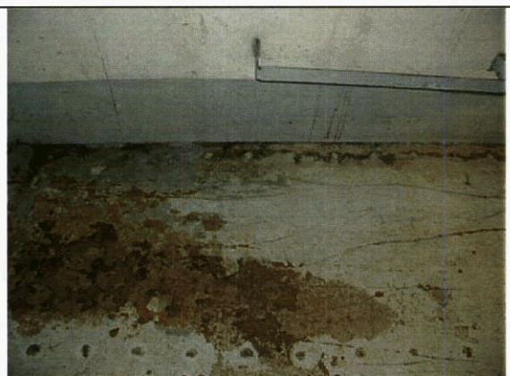
Figure 5.2B Broom clean on a painted deck. Note that rust need not be removed.
