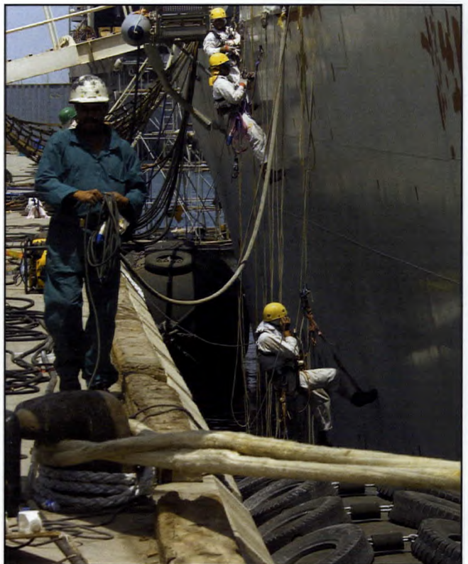
Routine maintenance, such as these touch-ups to Fredericton's hull, were arranged by the FLS staff to coincide with ships' visits to Gulf ports. (HMCS Fredericton photo by Corporal Mike Selig, HS032540d06)
