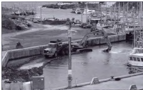
Harbour dredging at Port de Grave, Newfoundland. (Photo courtesy of Bill Jenkins, Small Craft Harbours branch, Newfoundland)
