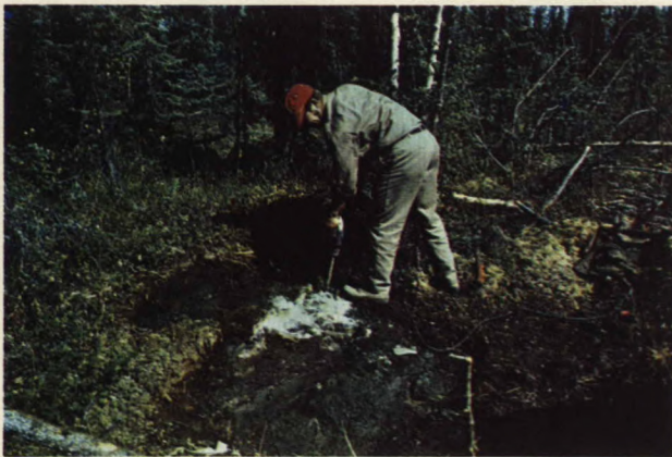
Figure 35. Digging highly icy near-surface perma- frost with an electrically powered jackhammer. Location: Lat. 65°47'N and 134°56'W
