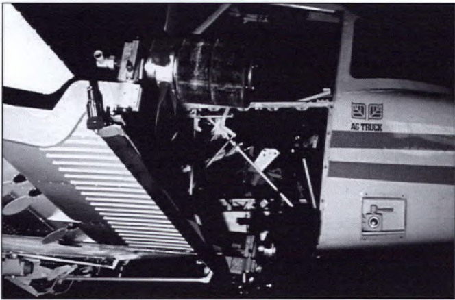
Figure 3. Micronair® AU3000 rotary atomizers installed on support booms in a Cessna-188 Ag Truck.
