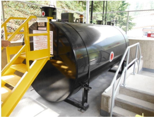
Petroleum Storage Tank for Emergency Generator, Kwikwexwelhp Healing Village, Pacific Region
