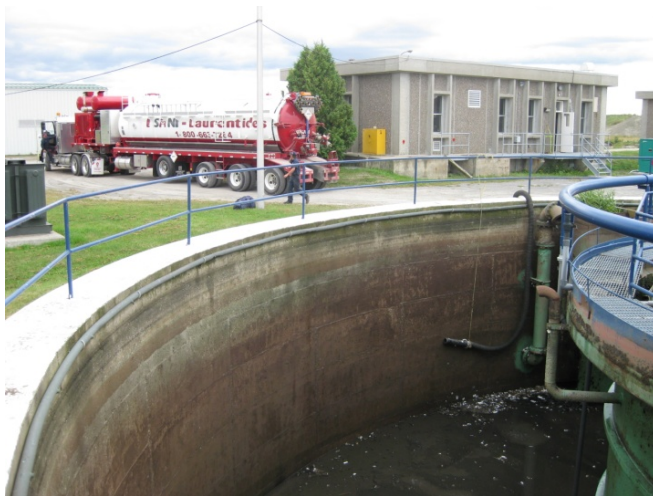
Wastewater Treatment Plant Sainte-Anne-des-Plaines – Quebec Region
