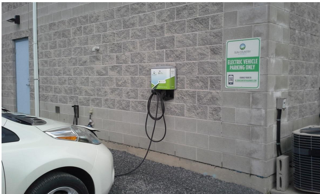
Electric vehicle and charging station at Collins Bay Institution, Kingston, ON.
