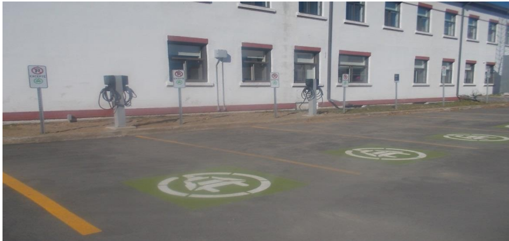
Electric vehicle charging stations at Regional Headquarters, Laval, QC.
