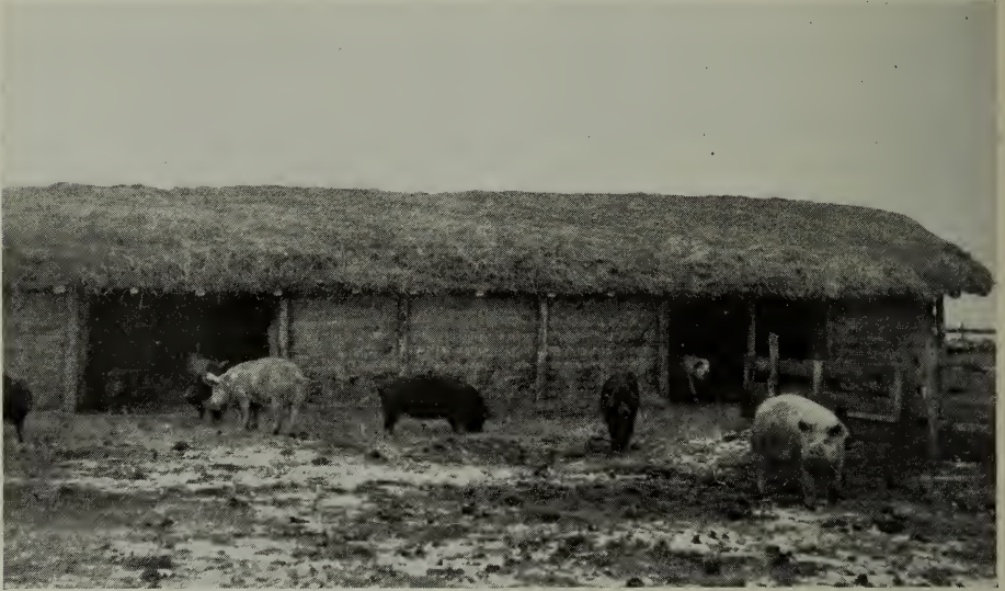
Straw shed completed. It was found necessary to fill in one of the doors in order to avoid drafts.
