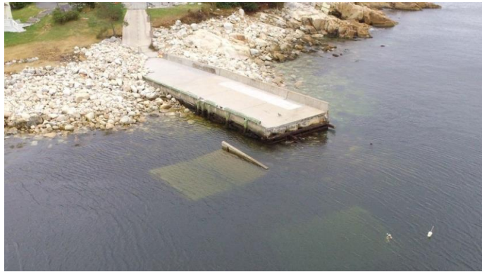
After Hurricane Dorian with 12 metres broken off and remainder damaged
