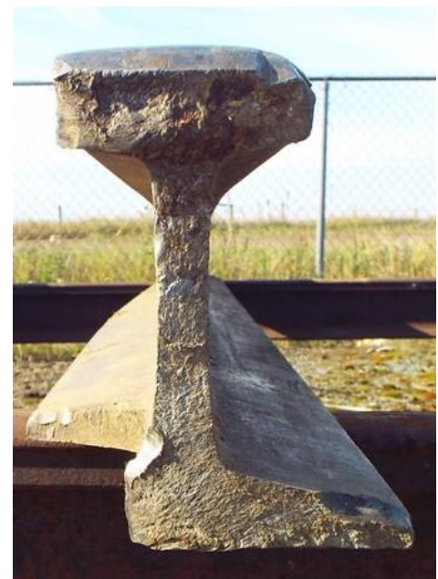
Figure 4. Broken rail showing rail end batter (Source: Canadian National Railway Company)
