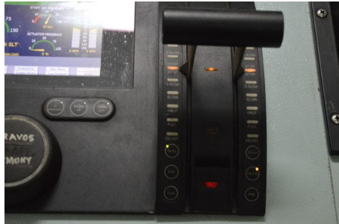
Figure 6. Combined lever and telegraph unit (LTU) on the Caravos Harmony (Source: TSB)
