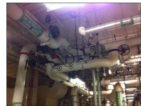
Cooling tower pipes in NRC building
