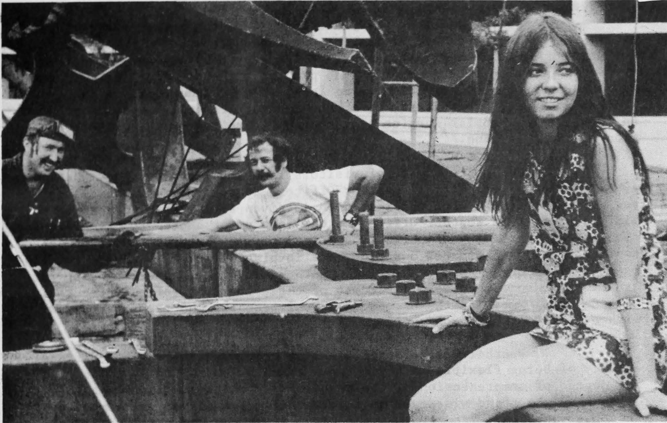
WORKMEN ERECTING a 110 foot sculpture by Ron Baird outside the new Atmospheric Environment Service Building in Downsview. York University student Carole Thompson stopped to watch. The sculpture is symbolic of meteorologists carrying weather-measuring instruments. Staff photo
