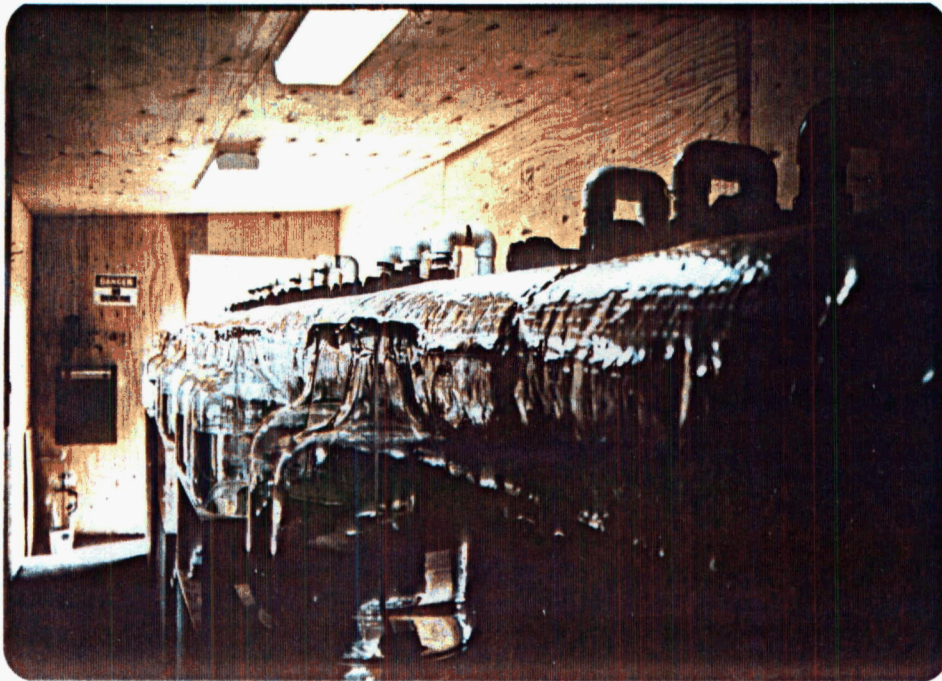
Figure 5. Interior of main shed showing the nutrient containers, the horizontal water distribution pipe (covered with reflective fibreglass insulation) and part of the water supply piping to each of the twelve mixing tanks.
