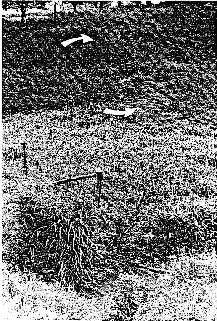
Plate 9. Another source of sediment noted in Skinner Brook just west of Weston is this waste water outflow indicated by the upper arrow. The other arrow points to deposits from the outflow.
