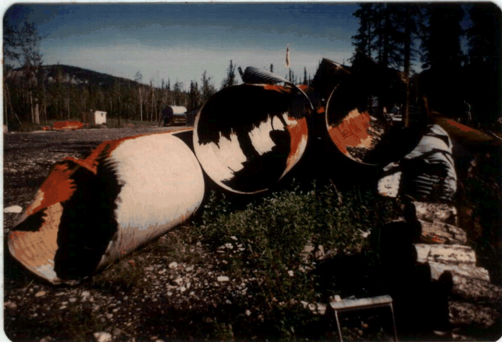
Plate 21. Corrosion of culverts after one year exposure to acid drainage
