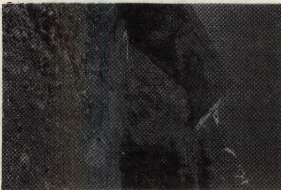
looking upstream (note washout of 8" dia. pipeline)
