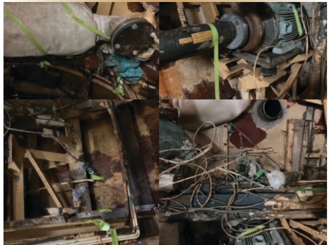
Figures 2a & 2b. The first hurdle was to finish removing the many interference items inside the ship that were blocking full access to the frames, longitudinals and hull plating.
