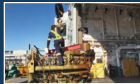
Staff from Fleet Maintenance Facility Cape Scott in Halifax remove the old MWM 602 diesel engine from HMCS Ville de Québec's after auxiliary machinery room. (Photo courtesy FMF Cape Scott)
