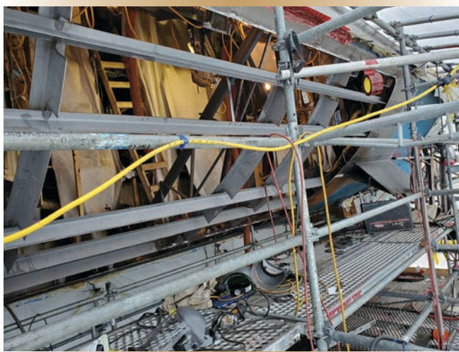
Figure 1. Scaffolding set up inside the weather enclosure, with the ship's side plating and section of angled bilge keel removed.
