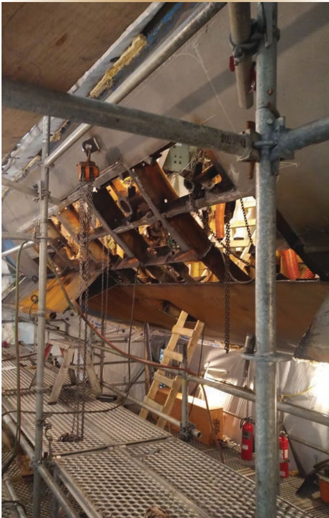
Figure 3. The 18-m 2 rectangular opening went from the after engine room (AER) to just inside the forward engine room (FER).
