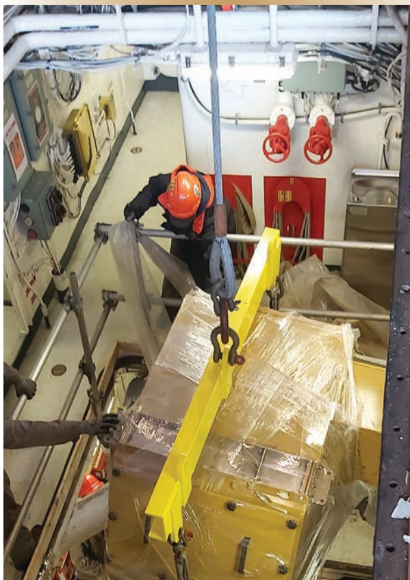
Figure 3a and b. A new Hitinger generator is moved through the ship's hangar, and lowered into the AAMR.
