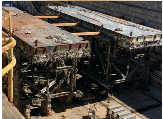
Figure 2. The substantial marine growth and murky conditions during the underwater survey hid the extent of work that would be required to fully repair the camels. In the end, the full cleaning and repair job had to be conducted across two separate docking windows.
