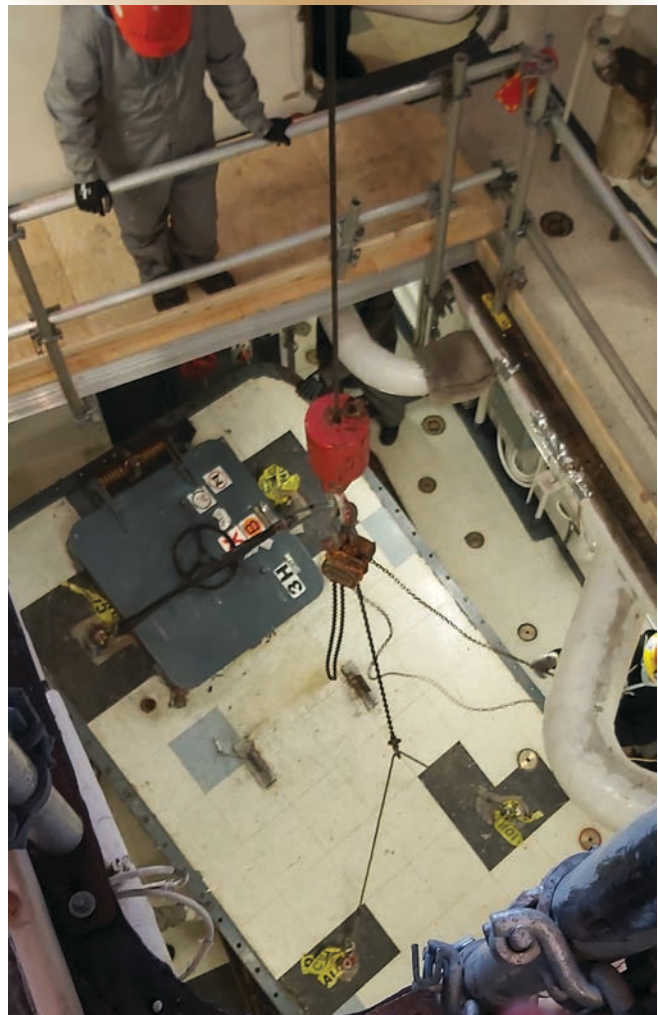
Figure 1. FMFCS personnel remove the soft patch into HMCS Ville de Québec 's after auxiliary machinery room (AAMR).
