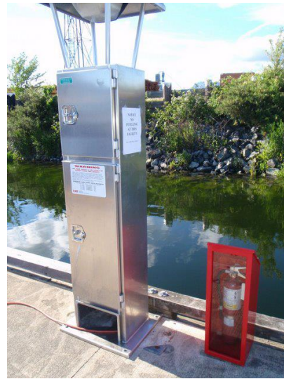
Power outlet distribution with breakers and lights fixture combined.
