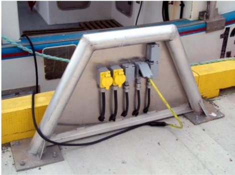
120V and 240V outlets
