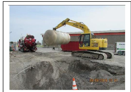
Underground petroleum storage tank Archambault Complex, QUE
