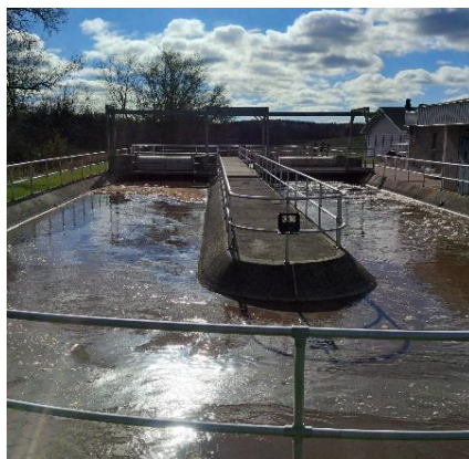
Wastewater Treatment Plant, Warkworth Institution, ONT
