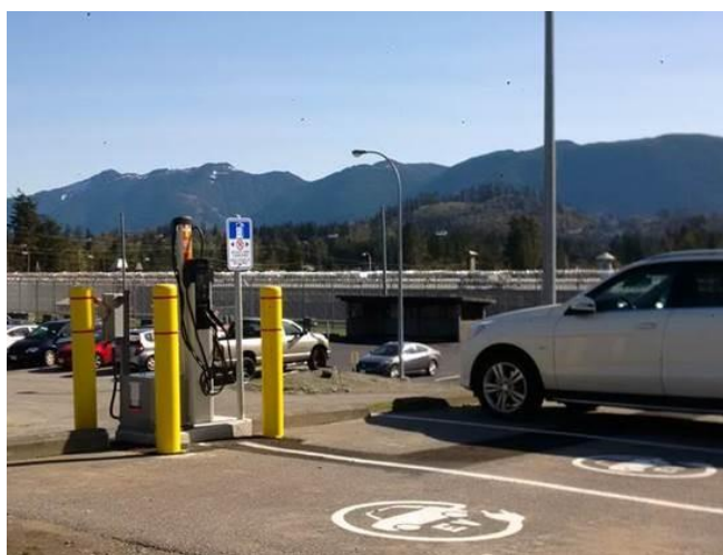
Electric Vehicle Charging Stations, Mission Institution, PAC
