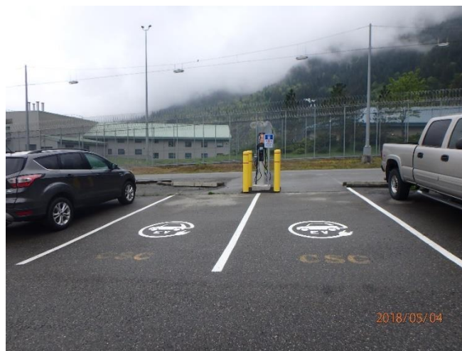
Electric Vehicle Charging Station, Mountain Institution, PAC
