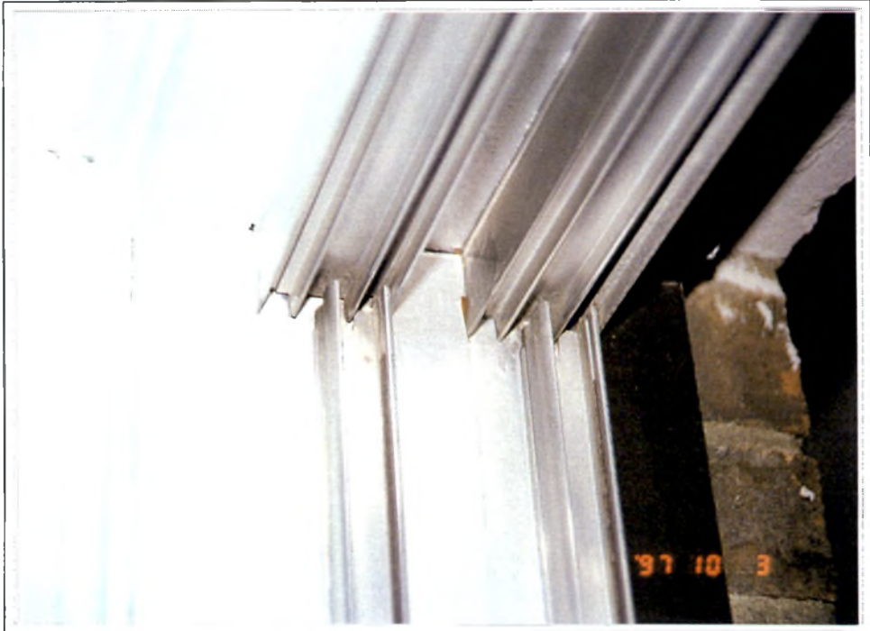
Photos #3 & #4: Views of head and sill condition showing the floating head track above and the weepholes at the sill track. Note the jamb weatherstripping which has dropped about 30mm permitting free air movement across the assembly.
