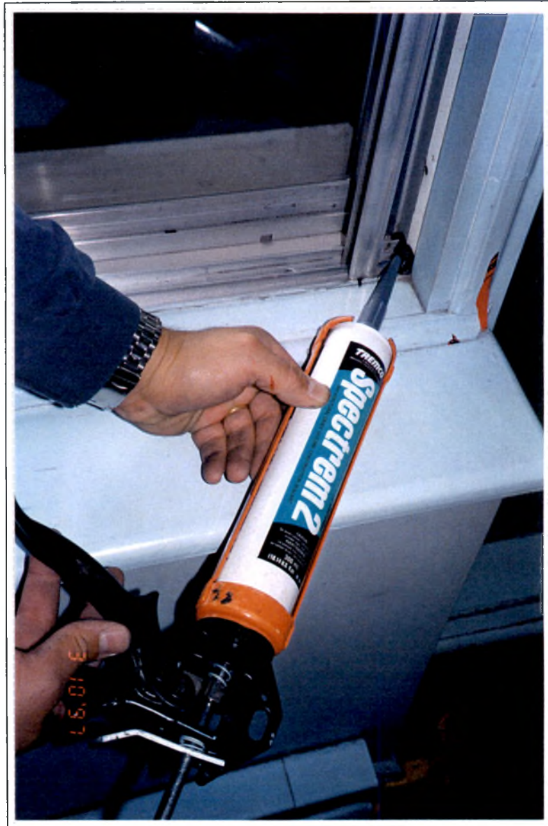
Photos #9: Application of caulking to seal the intersection of the jamb and the sill track at the L'Emminence apartments.
