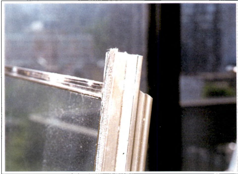
Photos #5: View of existing meeting rail weatherstripping at the La Cite Apartment test window.
