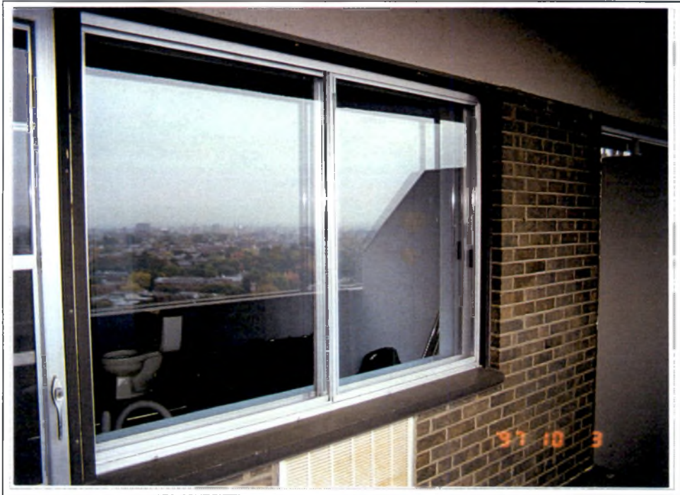
Photo # 1: Exterior view of aluminum sliding window at the L'Emminence apartment building. The unit is typical of the size and construction of the units studied.
