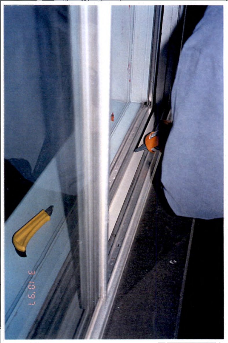
Photos #11: Application of caulking sealant at the perimeter of the interior window tracks and jambs.
