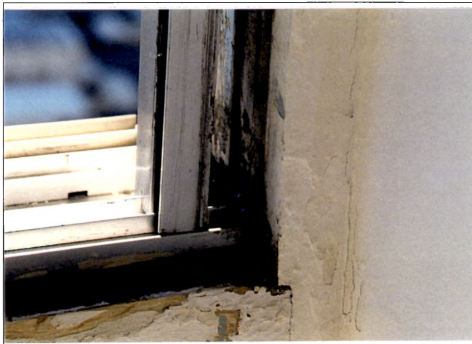
Photos #6: Existing sill/jamb condition at the St. Georges convalescent home. Note the severe deterioration of the wooden window frame due to prolonged water infiltration problems.
