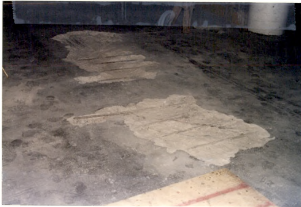
PHOTO B1: Typical delamination along the plane of top rebar in a parking structure slab.
