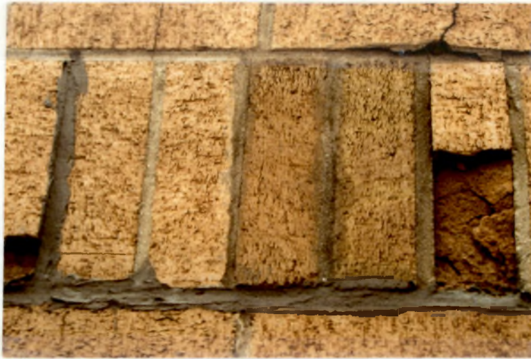
Fig. 3 Freeze/thaw damage at soldier course
