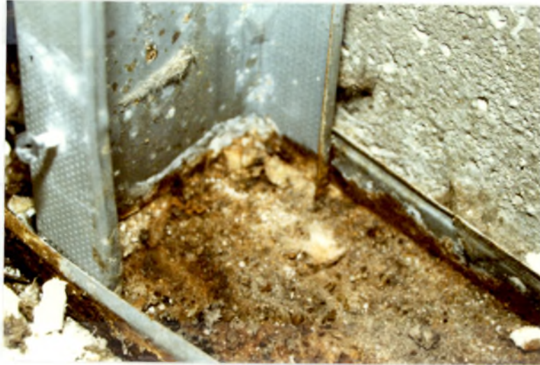
Fig. 11 Bottom track corrosion as seen in St. John's, Toronto and Calgary
