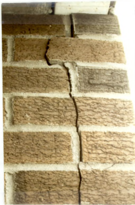
Fig. 4 Vertical cracking due to unintentional load transfer at balcony
