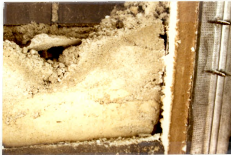
Fig. 8 Extensive mortar droppings at floor levels
