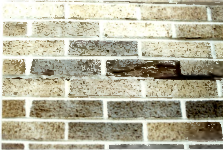
Fig. 5 Spalling of brick units at shelf angle location due to lack of a "soft" joint
