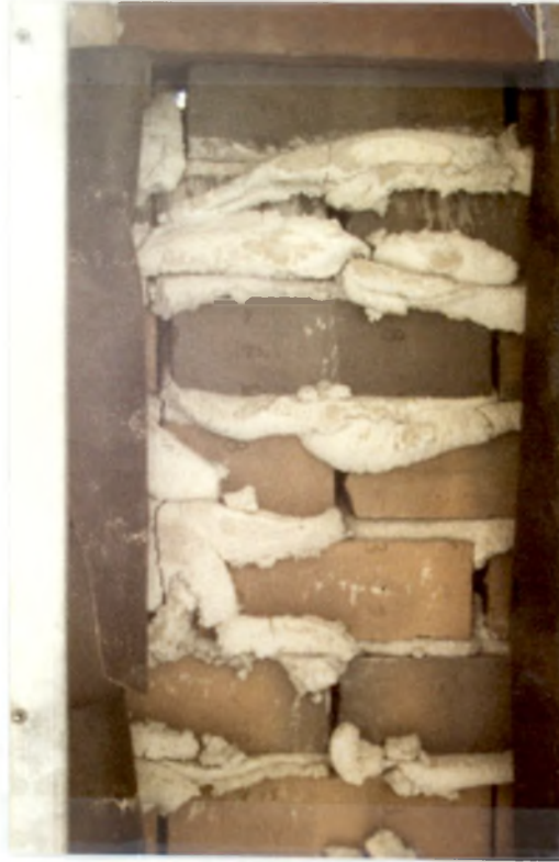
Fig. 7 Extensive mortar protrusions and poorly filled head joints.
