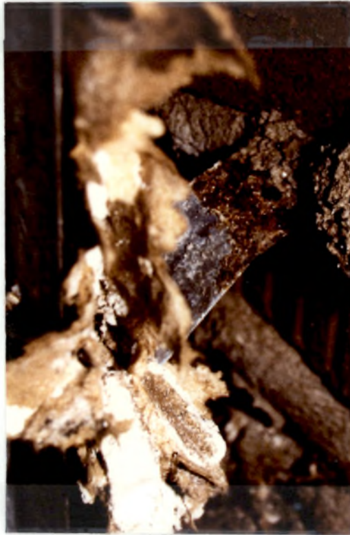
Fig. 10 Showing corroded strip tie after removal of mortar droppings
