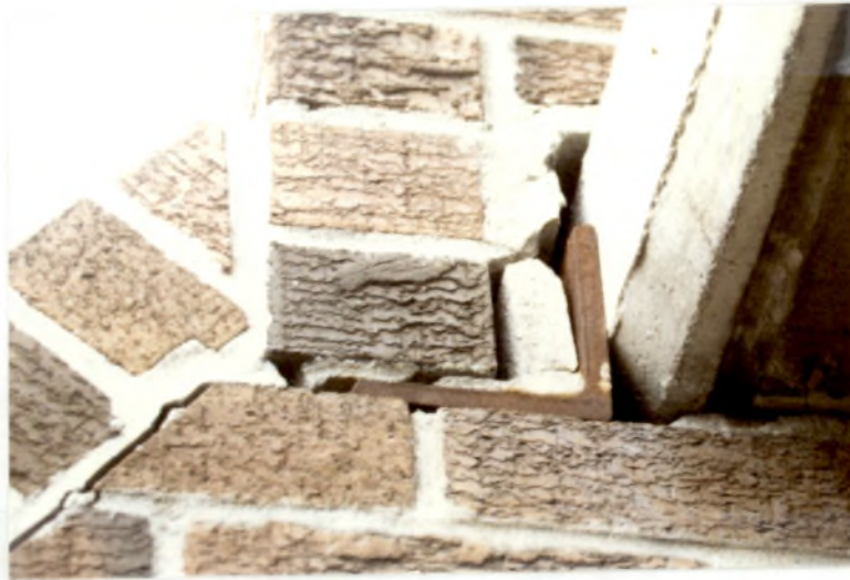
Fig. 6 Cracking of masonry due to poor detailing at balcony slab locations
