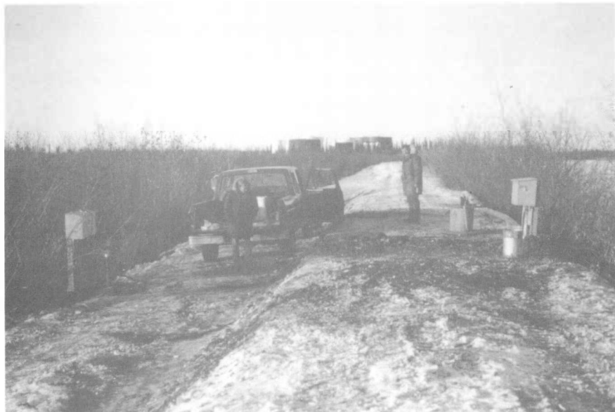
Photo 2 The Inuvik lagoon embankment, looking N.W., showing the completed termination boxes on both sides of the embankment.
